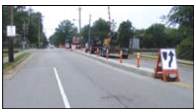
Geyer Road Left Turn Changes: Effective August 17, traffic can no longer turn left, or south, onto Geyer Road from Monroe. Southbound traffic on Geyer also can no longer turn left, or east, onto Monroe. Medians have been installed.
